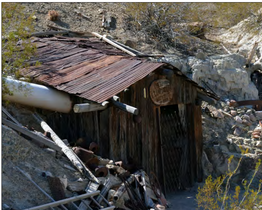
Figure 12. Old El Dorado Mine. Entrance to the underground mine tour. L.M. Vredenburgh photo Oct. 13, 2019.
